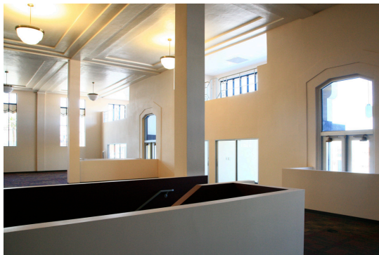
Main "high bay" space on the ground floor - subject to excessive reverberation.
